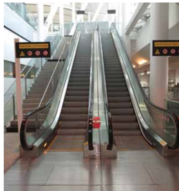
The CNIM escalators at Terminal 1 in Toronto Pearson.
