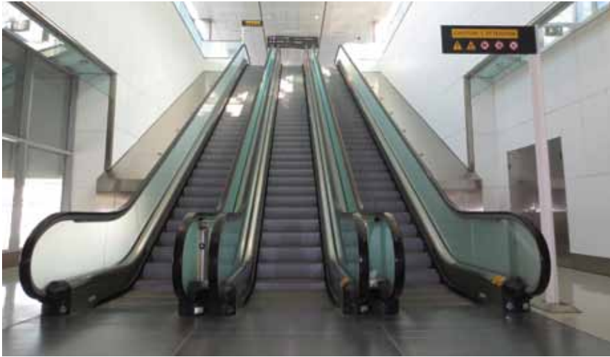
The ThyssenKrupp escalators at the Terminal 1 APM train station.
