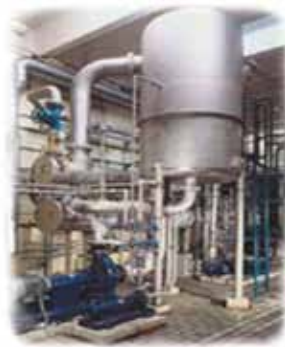
A pre-concentrator evaporation system.
