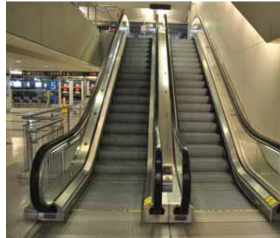
The ThyssenKrupp escalators at the Terminal 1 parking garage.
