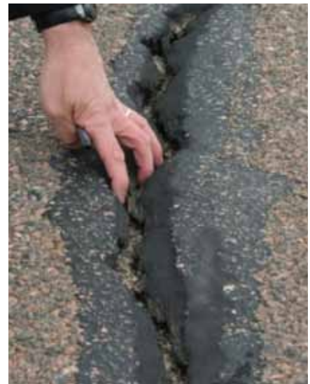
Before its facelift, the runway saw significant environmental degradation—a result of 27 years of service without major rehabilitation.
