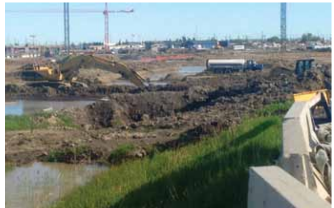
The concrete design requires careful planning and construction as Calgary has an ever-changing weather climate, making it difficult to construct the cement concrete runways and taxiways.
